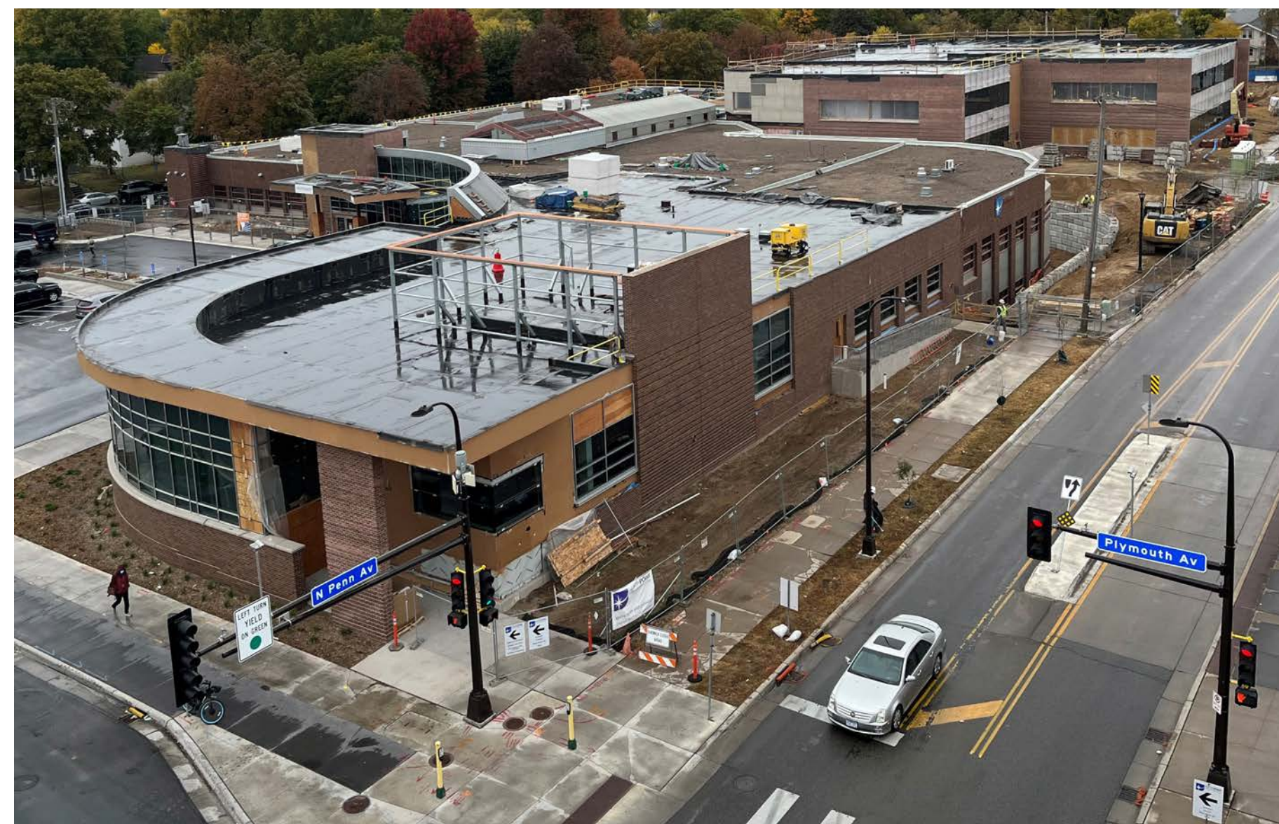
An aerial view of NorthPoint's main campus under construction from October 2022. Photo courtesy of NorthPoint Health & Wellness Center
